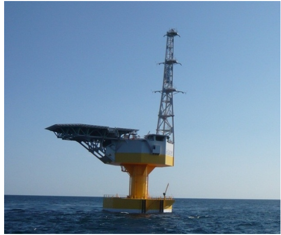
66kV Floating Substation “Fukushima Kizuna” (Floater: Advanced Spar)
